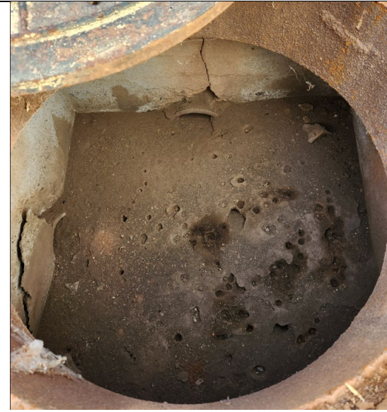
Photo 4: (05/06/2025) Manhole H-2 filled with sediment. Top of pipe barely visible top and left side of photo.
