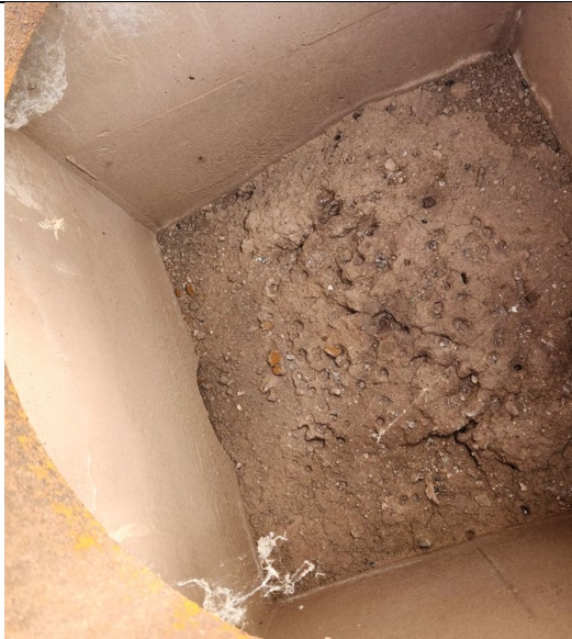
Photo 3: (05/06/2025) Manhole H-1 filled with sediment. Top of pipe entrance is barely visible on left side.
