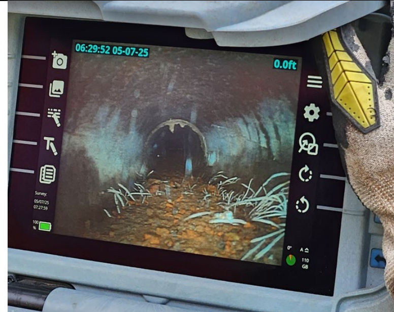
Photo 10: (05/07/2025) Root intrusion identified on field screen at manhole E-11.
