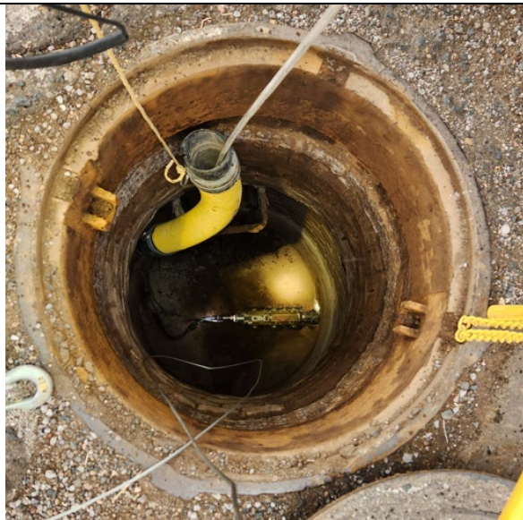
Photo 7: (05/07/2025) Manhole E-6 with 6" crawler camera deployed. Unable to bypass sediment at pipe entrance.
