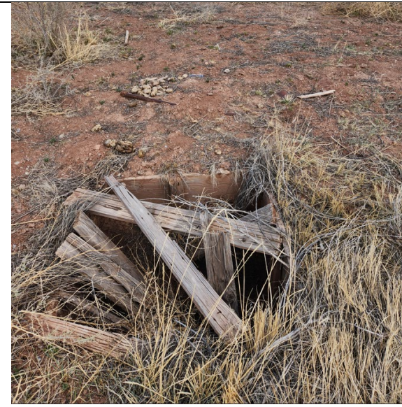
Photo 12: (05/08/2025) Collapsed manhole F-16.
