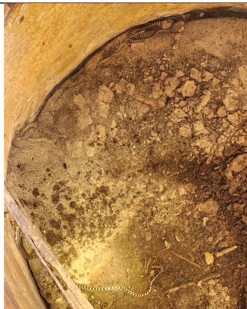
Photo 14: (05/08/2025) Manhole E-12 with sediment intrusion blocking E-W sewer lines access pipes. Two snakes found in manhole.
