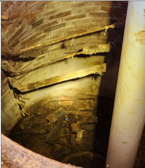
Photo 11: (05/08/2025) Damage inside manhole E-9 towards E-12.
